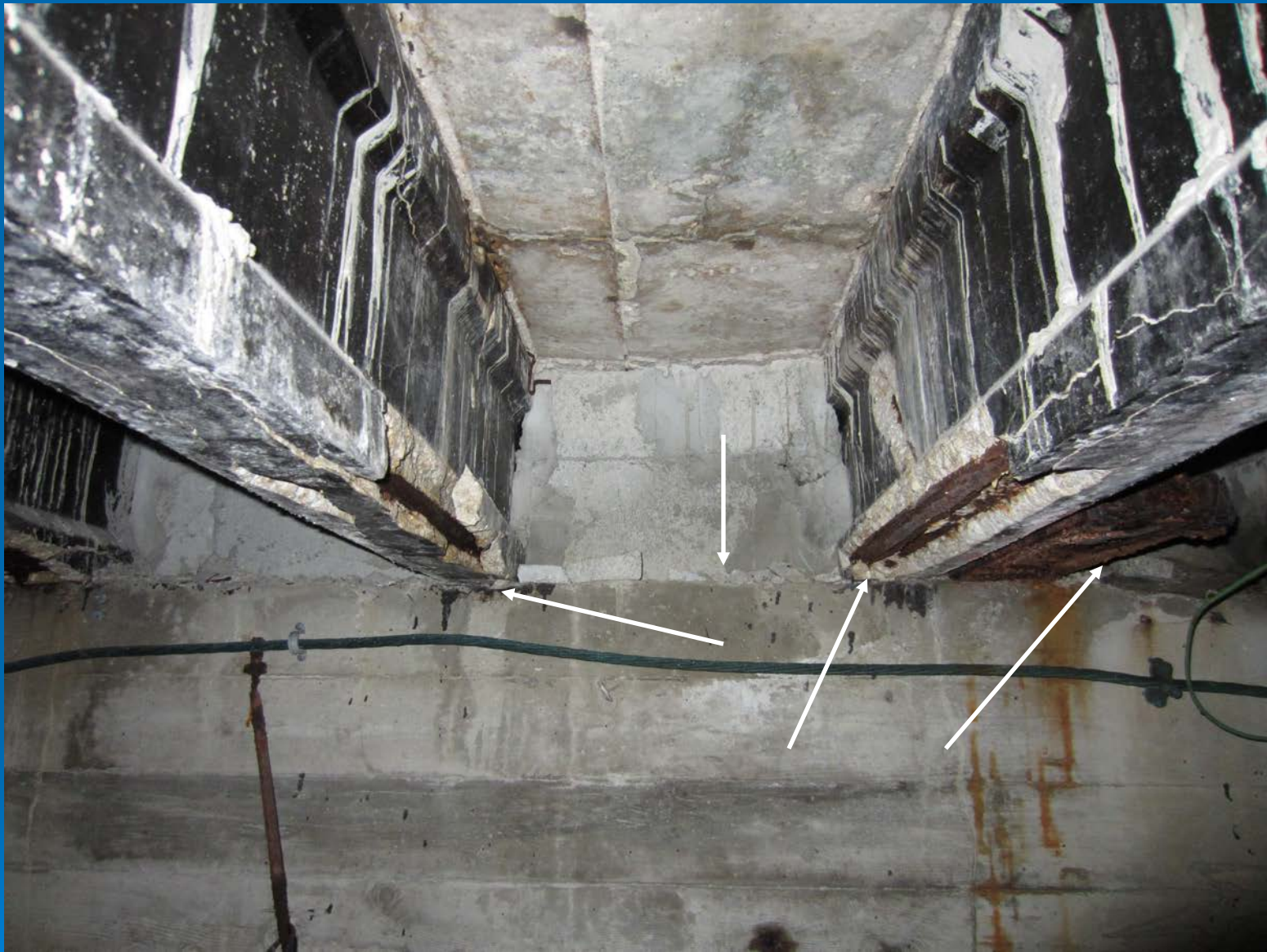
2 beams on either side have settled on top of the support-bearing beam due to the bottom steel breaking away the support edges
