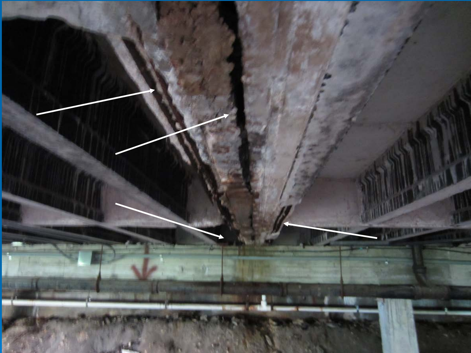
Expansion joint between 2 slabs perpendicular to the pool, west edge of slab being overstressed by I-beam
