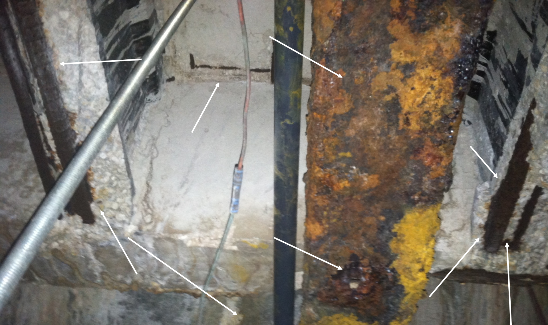
I- beams have lost their entire support of the upper deck due to structural steel corroding, expanding and breaking away the entire beam bottom. Note the drainage from the deck drains has totally corroded the waste pipe, allowing all rain water to flow on the ground, flooding area beneath the pool deck. This is black iron that was used in the 50's, as opposed to the PVC used today.
