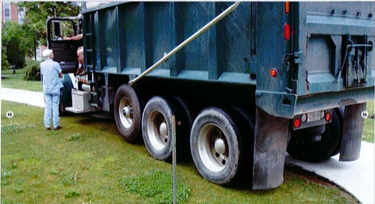
A loaded dump truck tests the strength of the Geoblock porous pavement system placed along the roadway to reduce rutting and turf damage.
