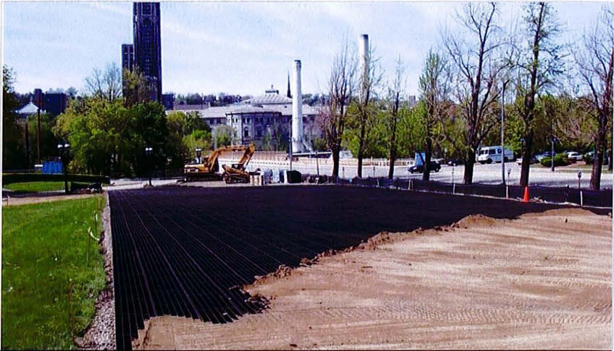
Installation of the Geoblock porous pavement system for a grassed overflow parking area.
