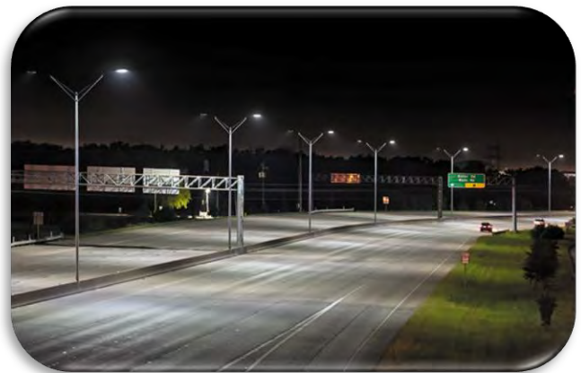
Proposed LED Fixture Installed in Baytown, TX
