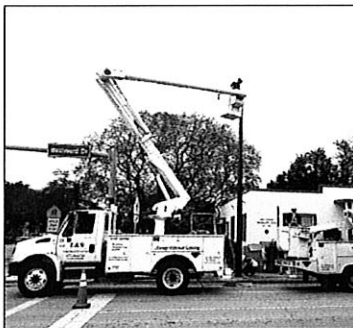
Contractors are installing 34 new decorative street lights and poles along Westward Drive. This is part of an ongoing City conversion to LED lighting to save energy and money.
