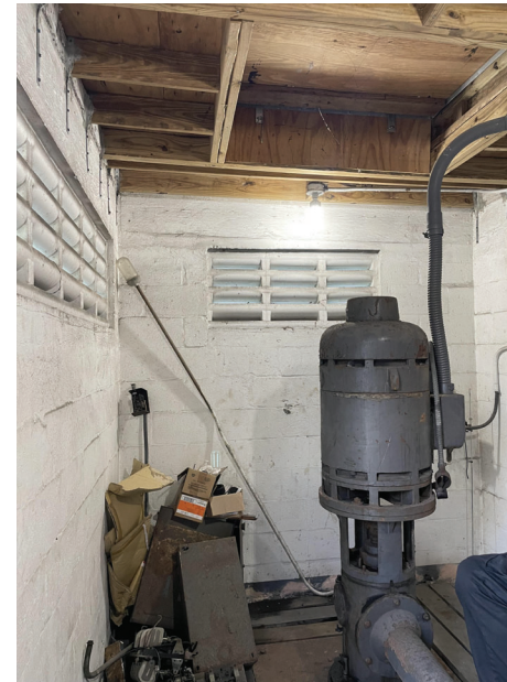
WATER PUMP STATION
